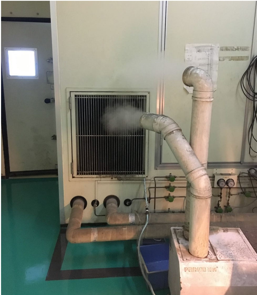
Fig. 1-2 Laboratory air return wall
